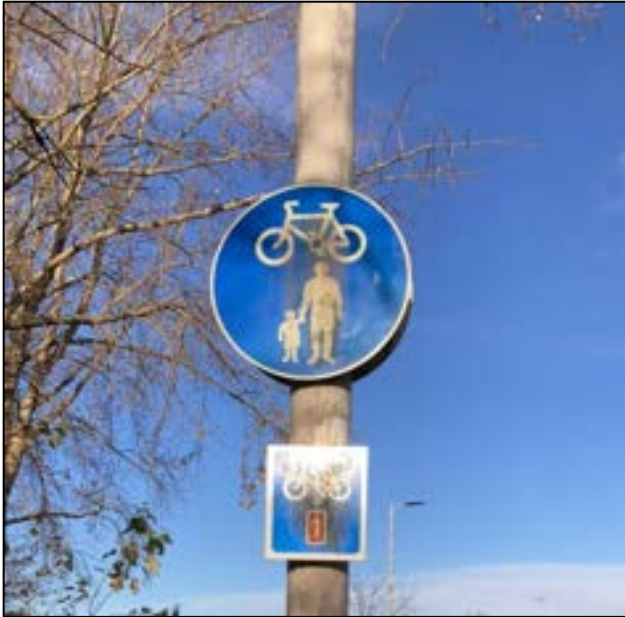
Figure 4 - Poor condition sign face example
