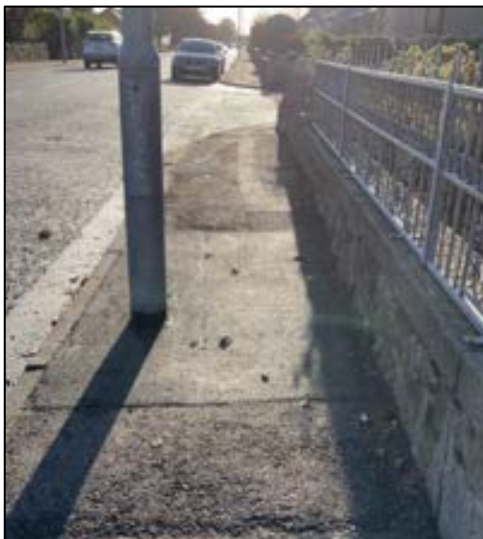
Figure 7 - Localised footway narrowing on Victoria Street
