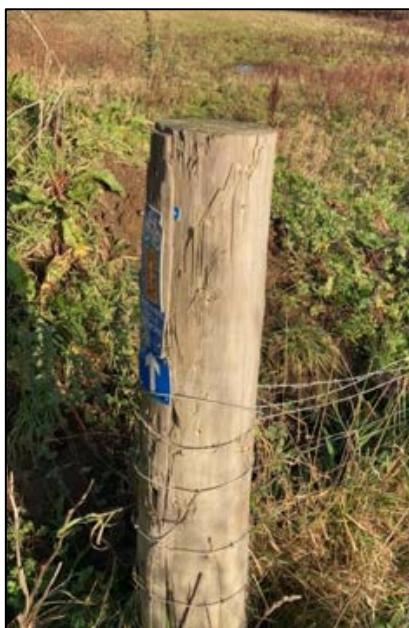
Figure 5 - Damaged wooden sign mounting post
