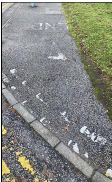
Figure 4 - Faded cycle markings on Wellheads Drive footway
