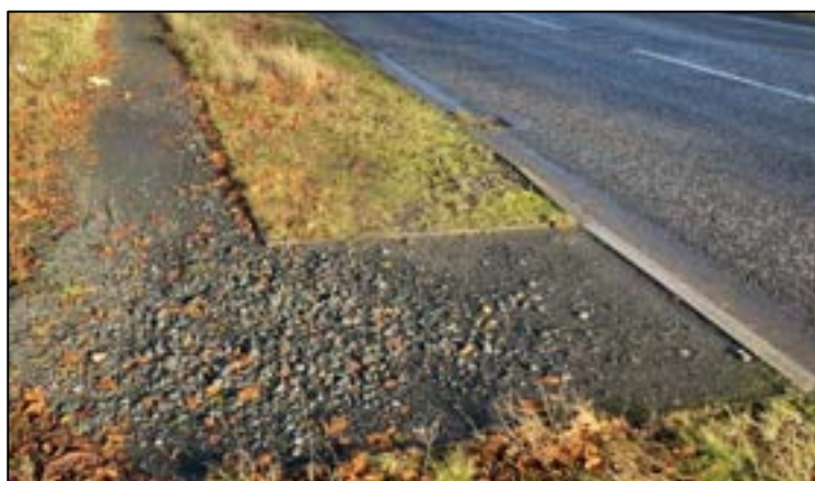
Figure 6 - Example of poor footway condition on Old Meldrum Road
